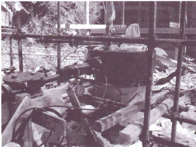
Figure 4. Collar on pile n° 3.
