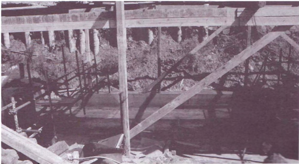
Figure 11. Components of the test device between pile n° 1 and pile n° 2; starting from pile n° 1 are visible the quick release device, the CROSBY turnbuckle, the load cell and the steel rope passing over pile n° 2. The support structure for the displacement transducers is also visible in the vicinity of pile n° 1.
